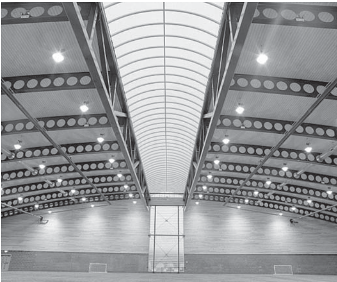
Fig. 1.12 Cellular beams over Rangers FC, an indoor training facility in Scotland (Courtesy: ASD Westok Ltd, UK)
